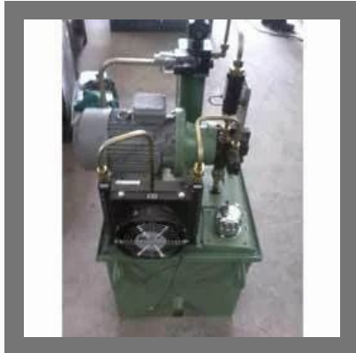
Power Pack Unit
